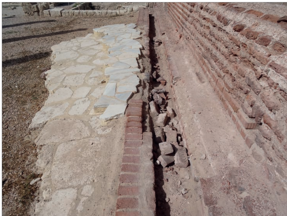
Fig. 11. The southern elevation of the bath, showing the damaged water channel (PCMA UW Alexandria Kom el-Dikka Project | photo G. Majcherek)
