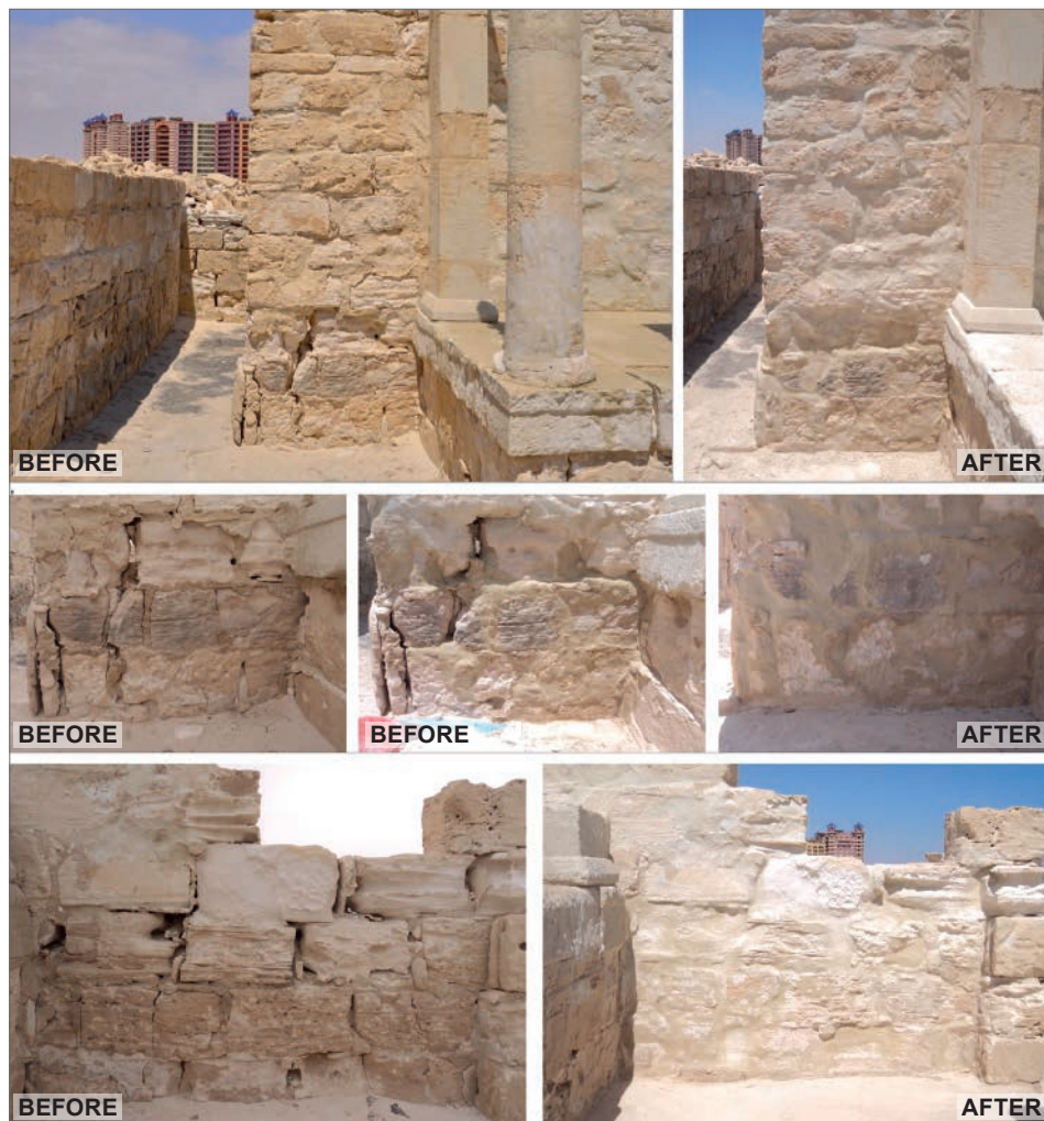
Fig. 8B. Commemorative monument before and after commencement of work in the 2018 season: details of the wall (Polish–Egyptian Conservation Mission | photos W. Grzegorek)
